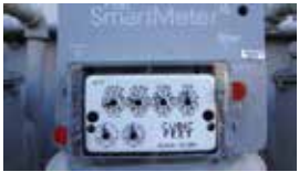
Automated Meter Reading
