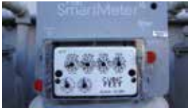
Automated Meter Reading
