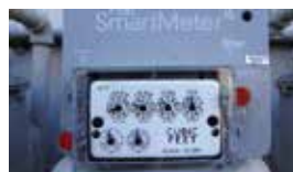
Automated Meter Reading
